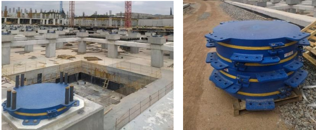
Figure 1.6. Aydın Şehir Hastanesi - AYDIN HOSPITAL isolation system
