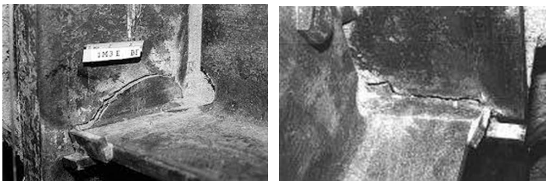
a. Column Flange "Divot" Fracture
