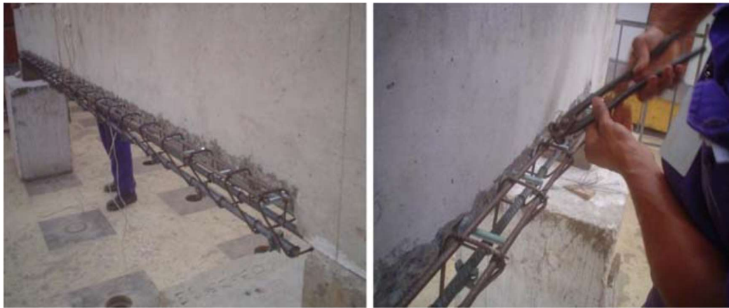
Figure 1.8. Fixation of the strengthening steel cages on the tensile side (Shehata, Shehata, Santos, & Simões, 2009)
