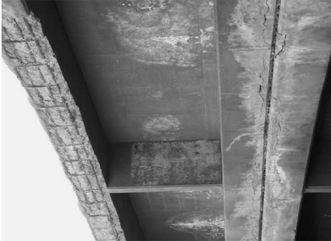
Figure 1.3. Example of steel corrosion (Chong 2004).
