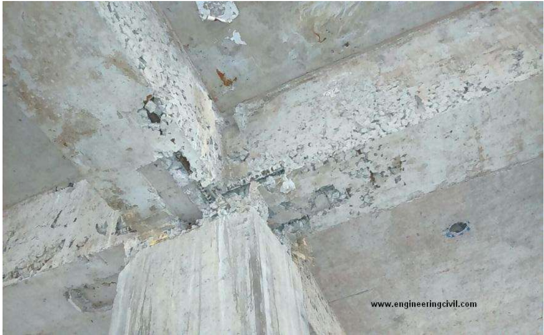
Figure 1.1. Faulty workmanship (Rogerson, 2018).
