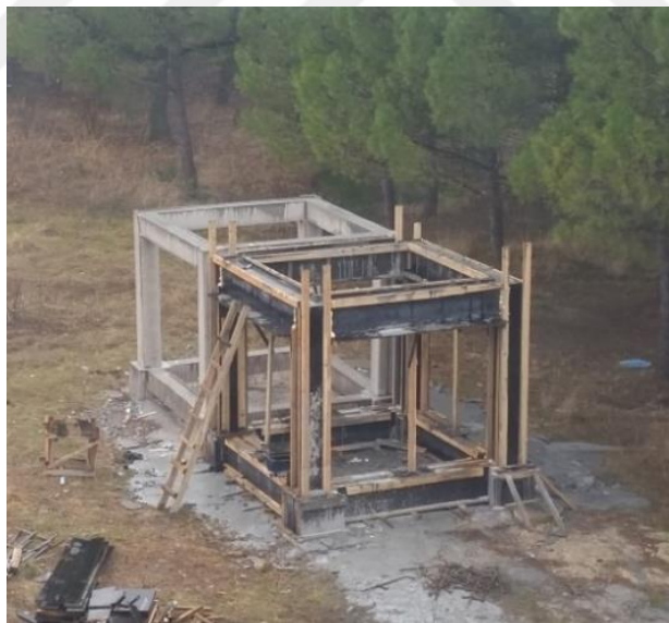
Figure 3.6. The working space of two frames when waiting for the age of concrete.
