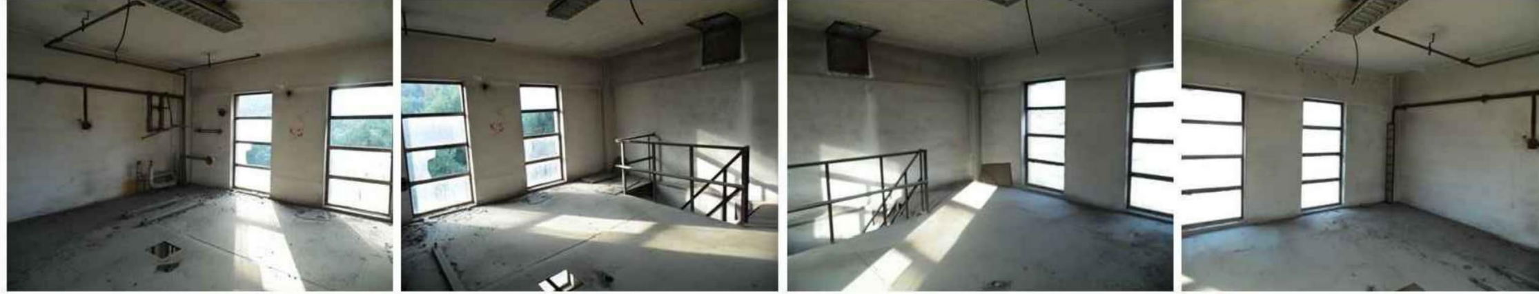
1.501 SOLVENT GERİ KAZANMA 2. 501 SOLVENT GERİ KAZANMA 3. 501 SOLVENT GERİ KAZANMA 4. 501 SOLVENT GERİ KAZANMA
